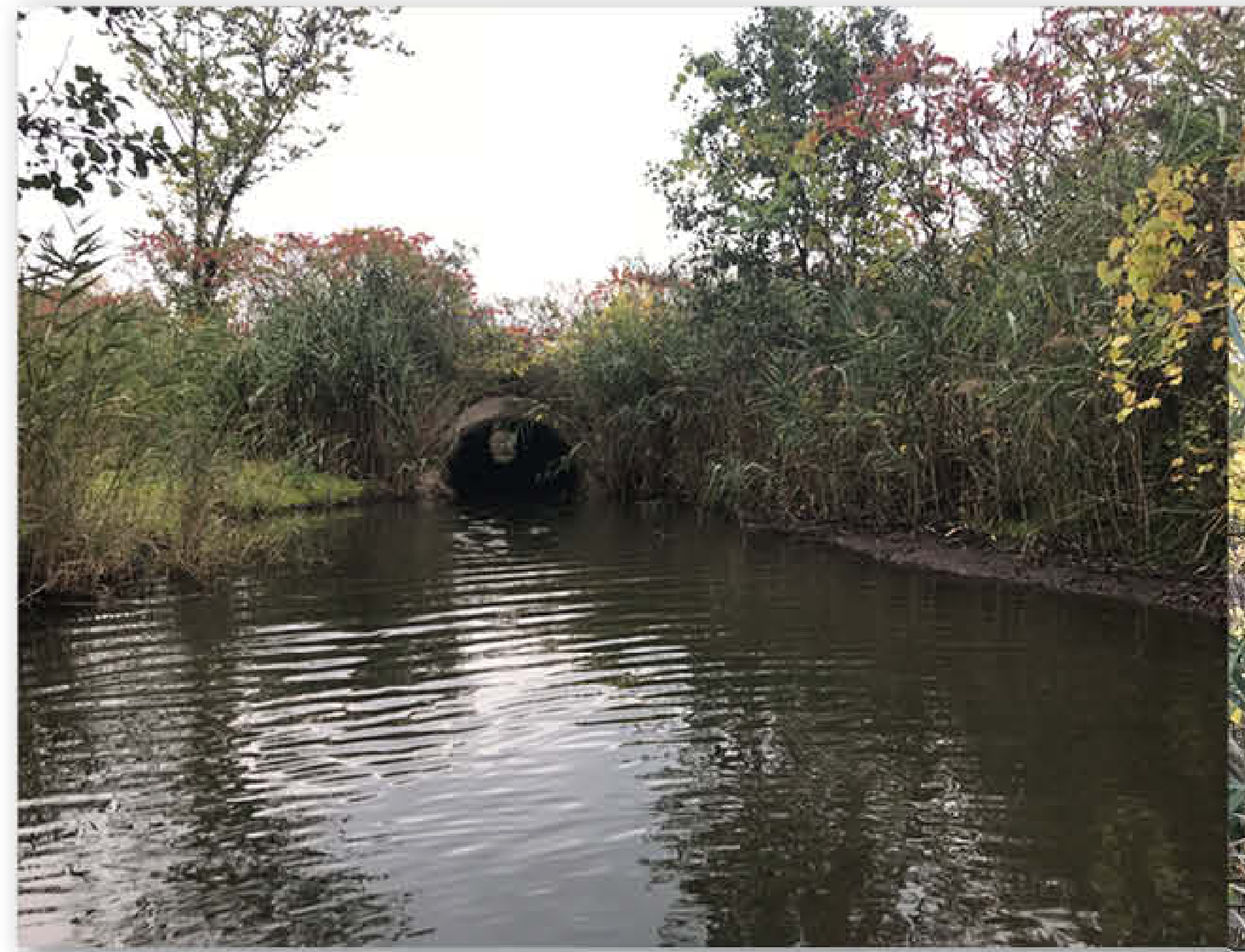
Outlet of culvert under NB & SB I-81 (future BL 81), north of NY 481
