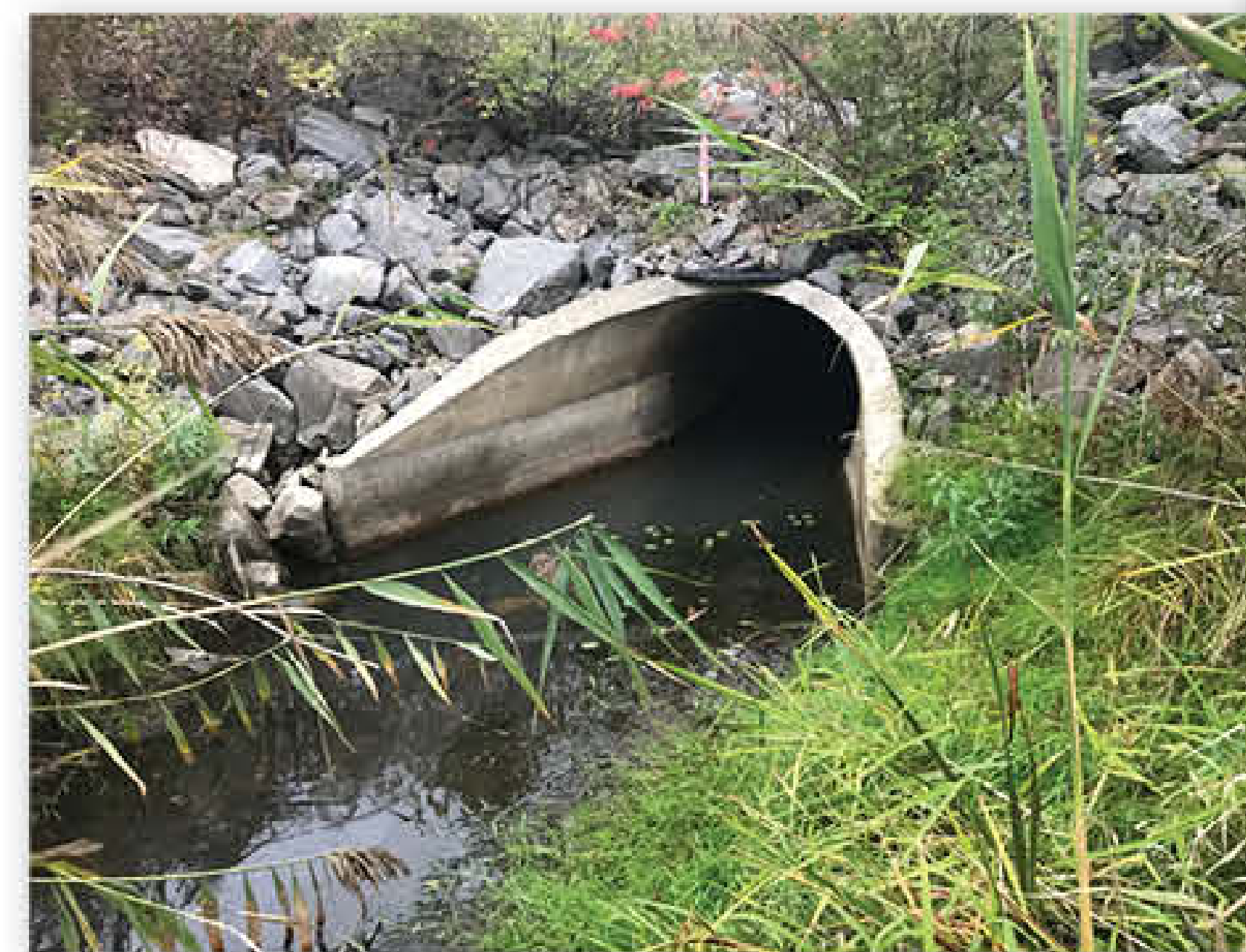
Outlet of culvert under NB & SB I-81 (future BL 81), north of NY 481
